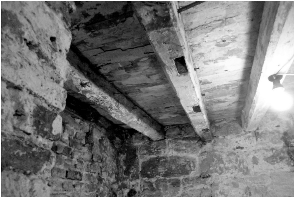
Figure 16: View looking east of beams 8 (the short one) and 2 and 3 showing evidence of re-use. The eastern ends of the beams sit on the masonry spine wall. The cross wall of 18th century brick is on the left.
