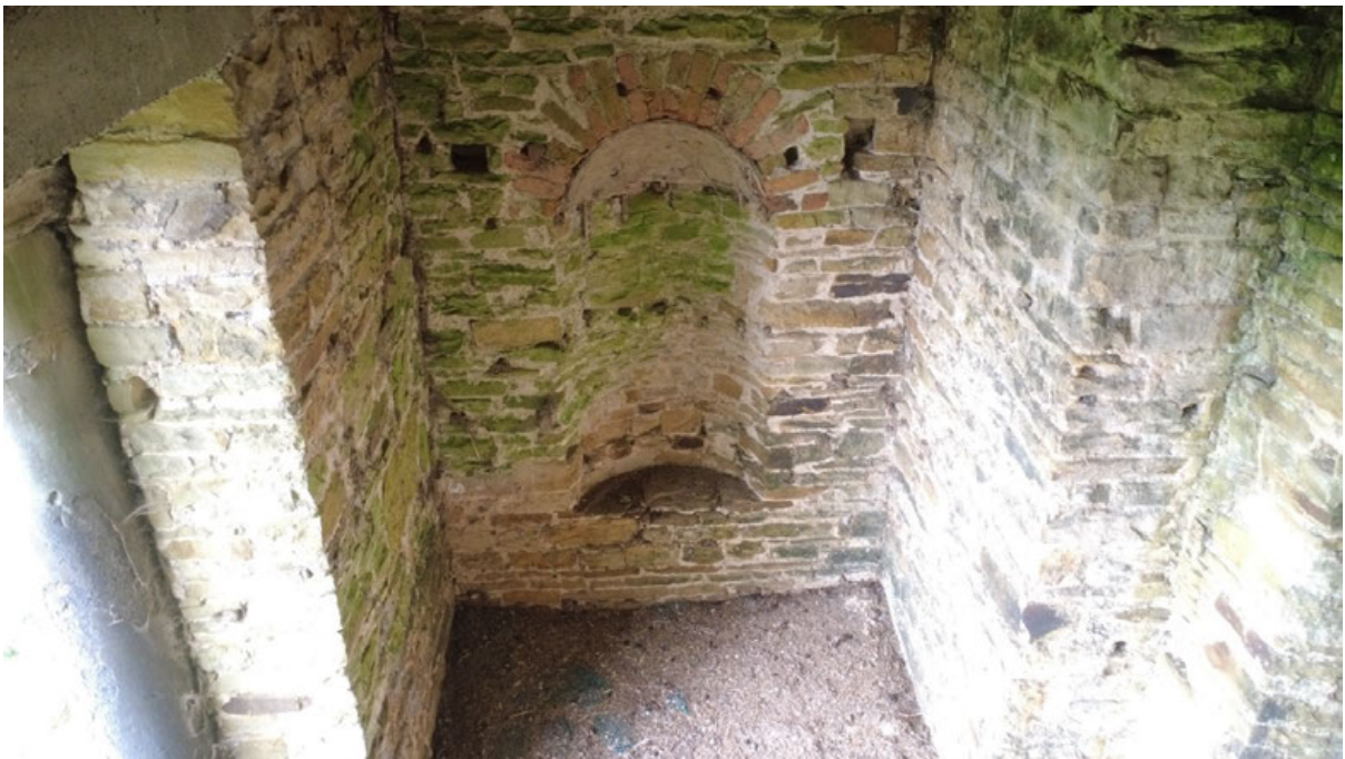
Fig. 32 Niche in the west wall. Note the brick-arch at the top and in situ lathe and plaster below. Holes for wooden plugs are visible within the niche and in the walls on either side indicating that the interior of the folly was probably plastered. (Photo by Mark Denton).
